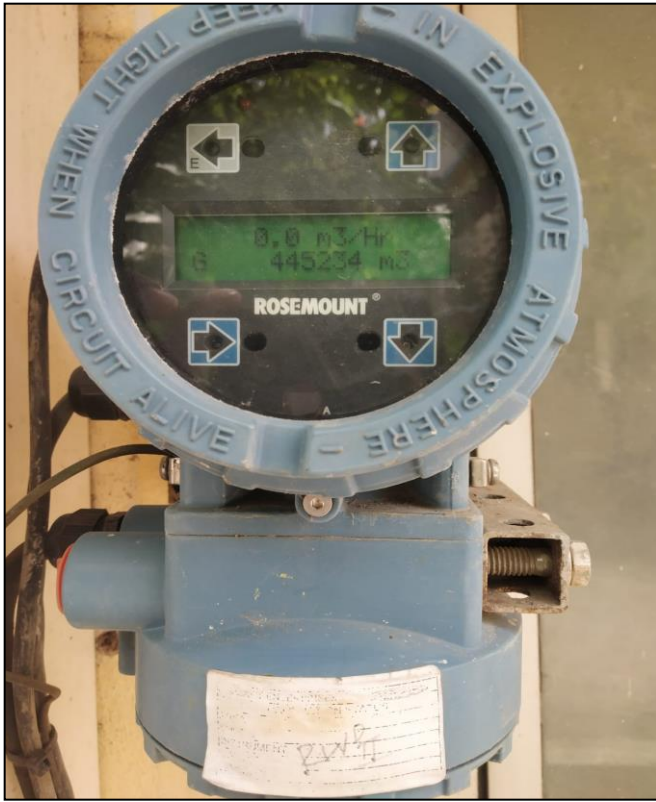
Inlet Flow Meter
