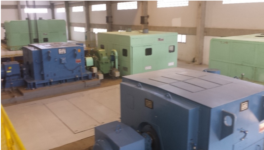
Power Generator 1, 2 and 3
