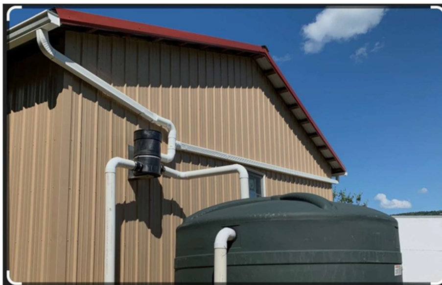
Figure 13.1: Rainwater Storage Unit
