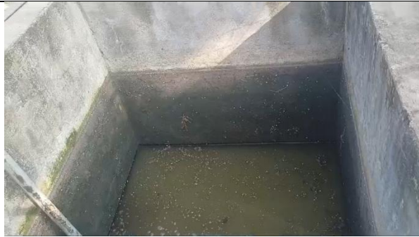
Sewage Water Collection Tank
