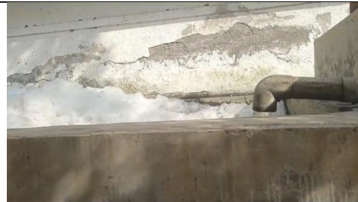
Bio Reactor / Aeration Tank
