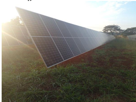
Image 1. Nova Ponte's PV modules.
